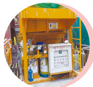
A wastewater reuse system on site
