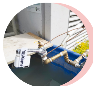
Water taps with motion sensors are installed on sites
